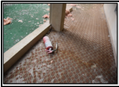
Several Extinguishers Used throughout
