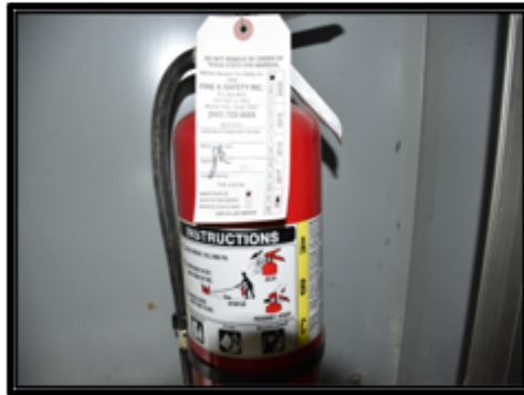
Improperly Maintained Extinguishers
