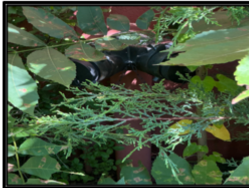
Fire Dept Connections hidden by growth July 2025
