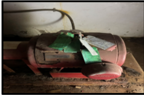
Corrosion on Fire Pump
