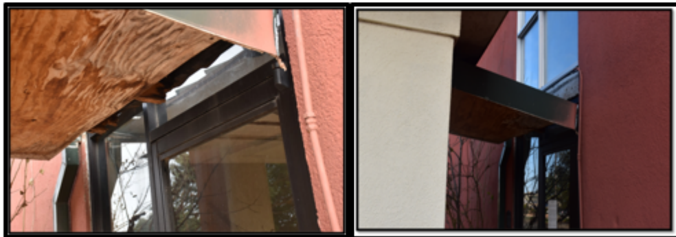
Photos of Northwest egress, walkway covering separating from structure
