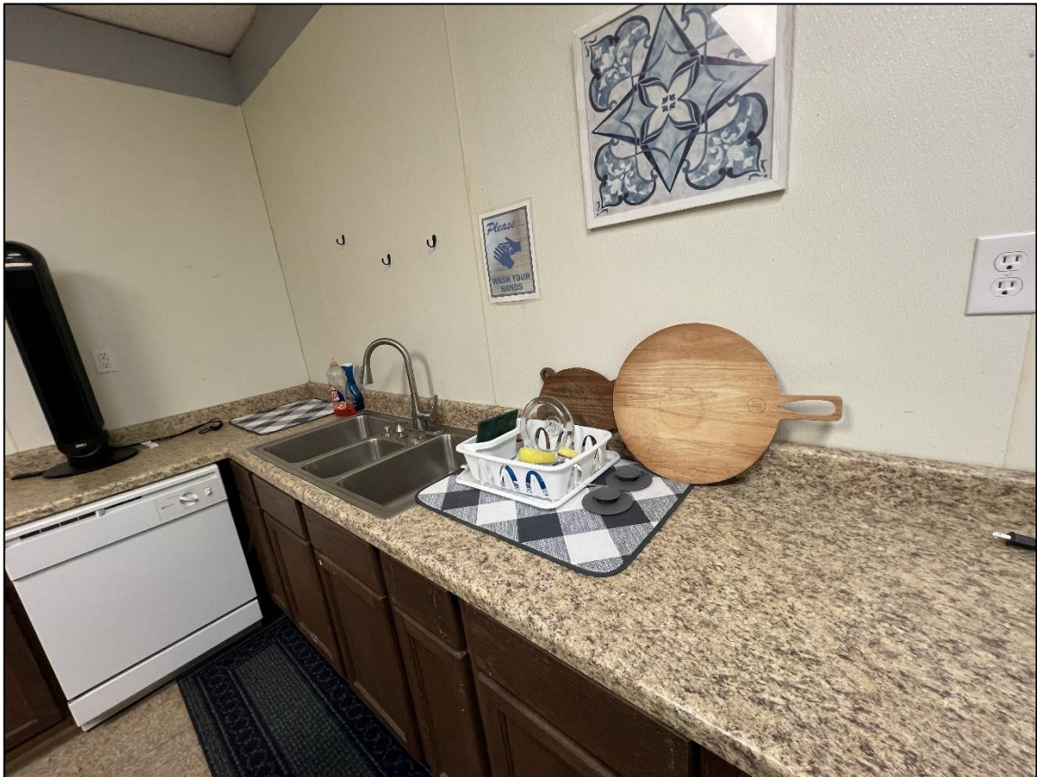
Project Photos Cont'd: 511 Mississippi (New Day Empowerment Center) Existing kitchen facilities; limited food preparation areas; ill-equipped and undersized.
